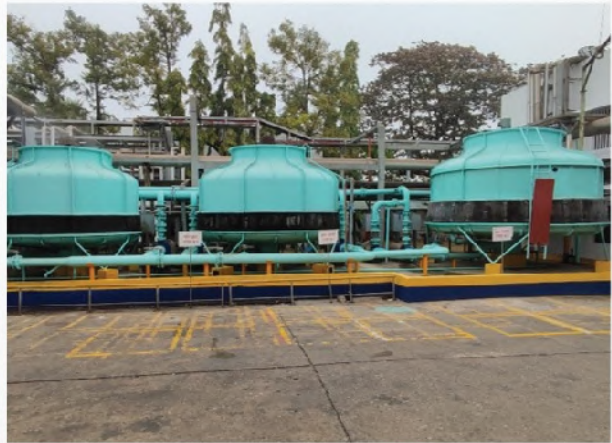
Seal Cooling water use in cooling Tower
