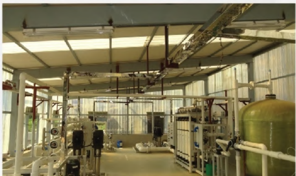
Reverse Osmosis(RO) plant
