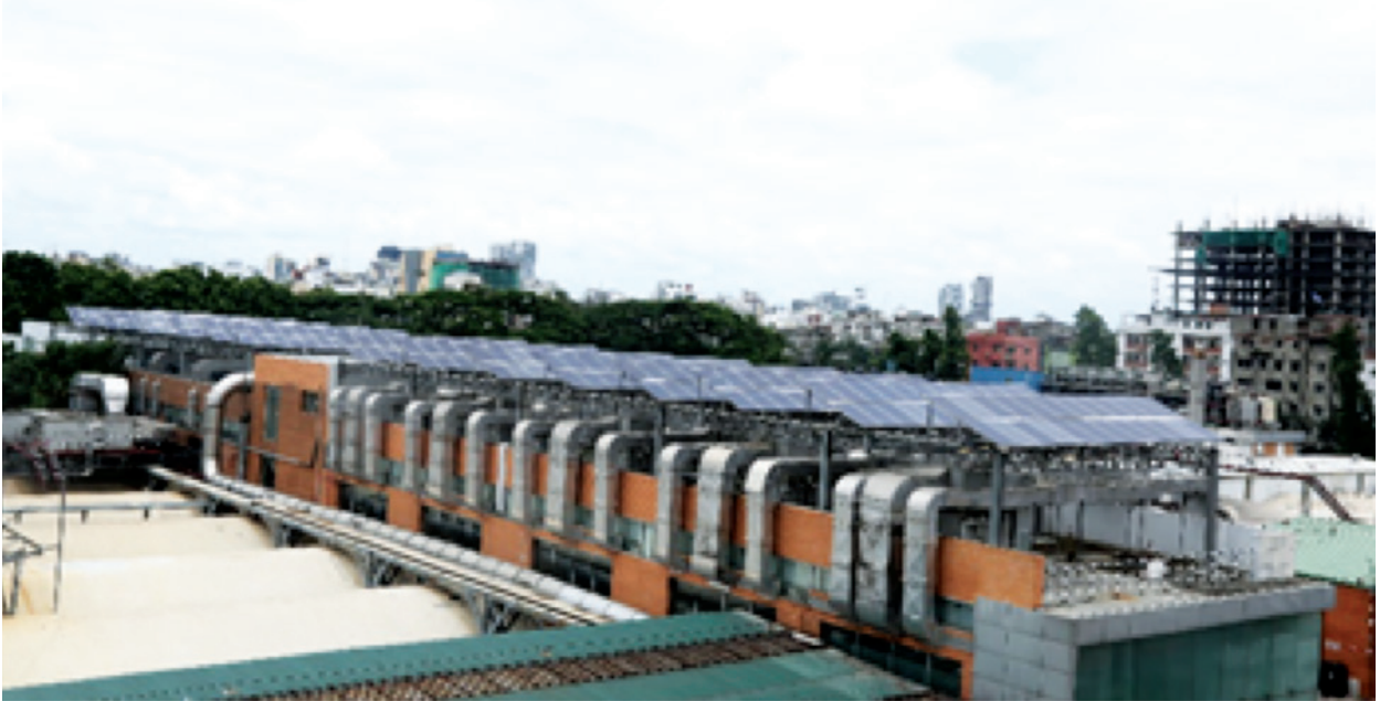
Solar panels installed to reduce electricity consumption
